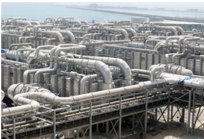
Marafiq MEDs with Steam and Vapor Ducting
